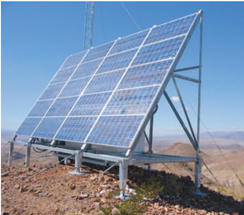
Multilateration Sensor with Solar Panel
